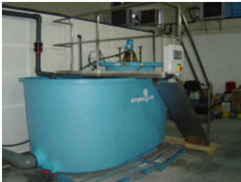
Skim in factory made tank (sump) in separate room from bins.
