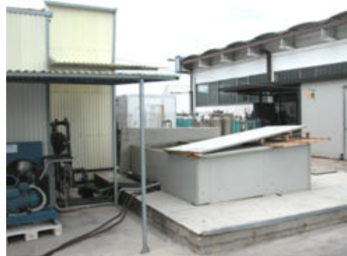
Skim in outside tank (sump) in separate location from bins.
