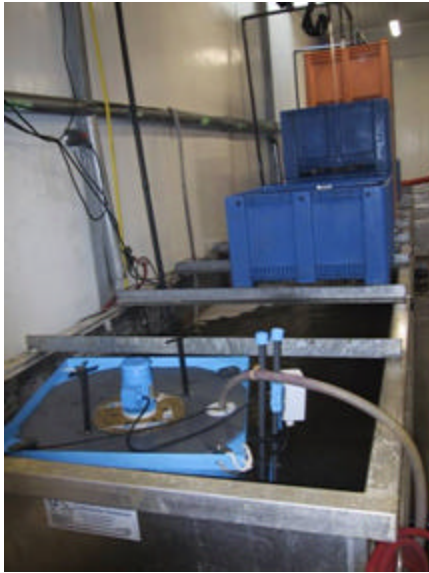
Centralized tank (sump) for bins and Skim.
